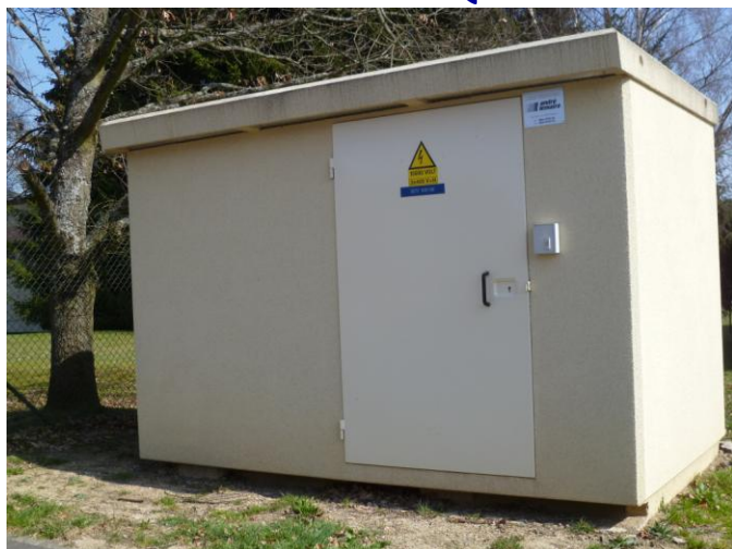
Cabine client "Roofland" à St. Vith.
